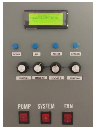
Figure 2. The control panel of the whole system
